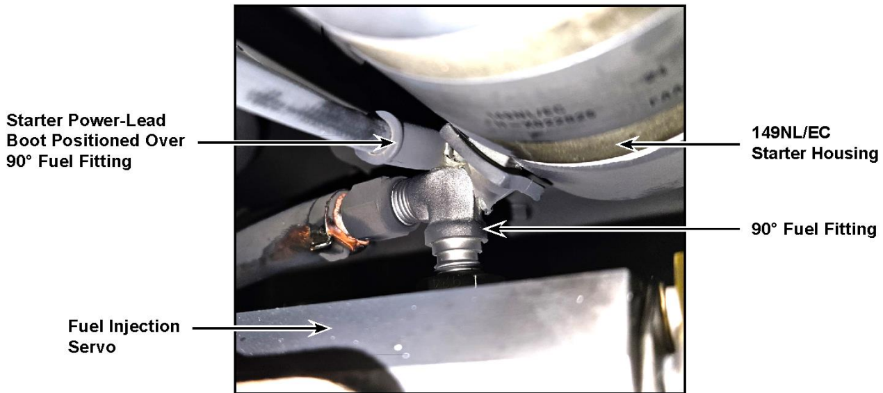
Figure-1 - Improper Starter Installation
